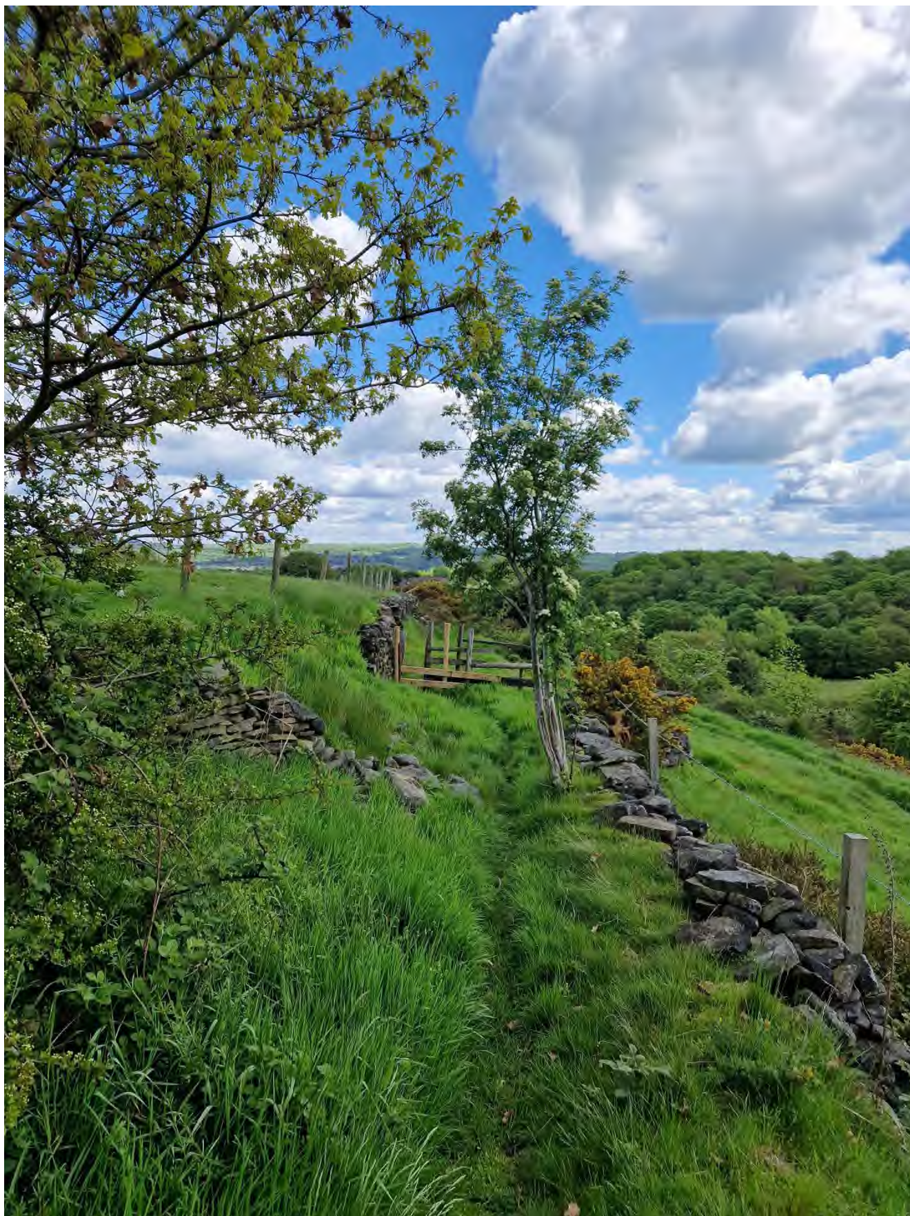
Photo 12: Second wooden stile structure limits the available width of the Order route at a point where the drystone wall on the southern side has collapsed (Grid Reference SE 1697 1258).
